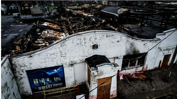
Photo of fire damage centering on original building 1
